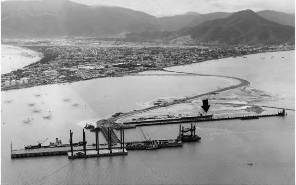
DeLong pier under construction at Qui Nhon in November 1966. Arrow indicates the hydraulic fill for port hardstand.
